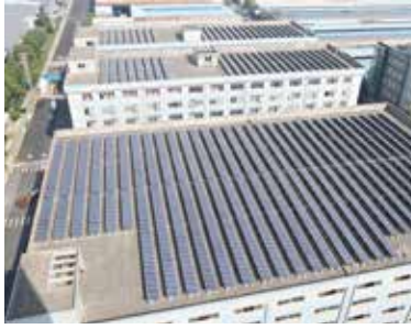
Solar PV Panels on the Roofs of Plants 廠區屋頂太陽能光伏板
